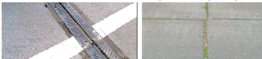
Figure 9.14: Gaps in roads and footpaths
